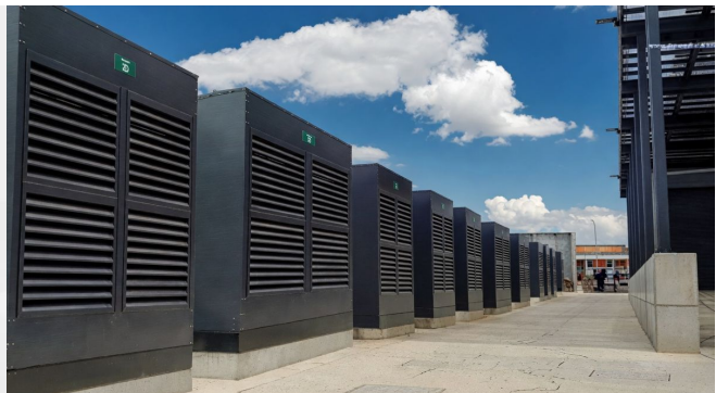
Row of FlexEgen acoustic enclosures — modular deployment at scale.
