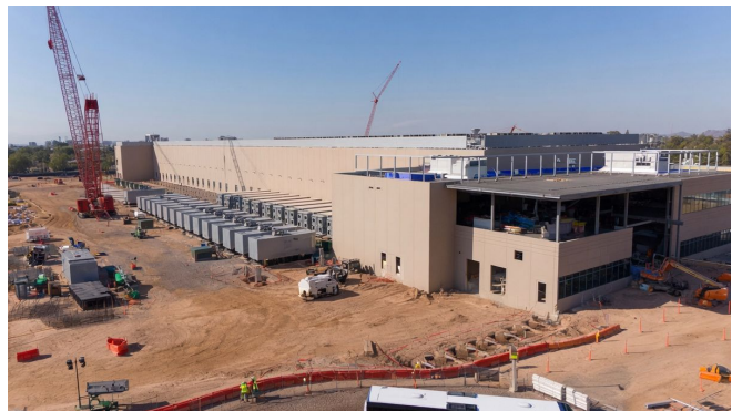
Modular cooling enclosures deployed alongside a live data centre.
