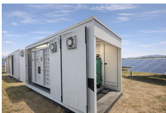
Deployed on a solar farm — modular switchgear enclosure.
